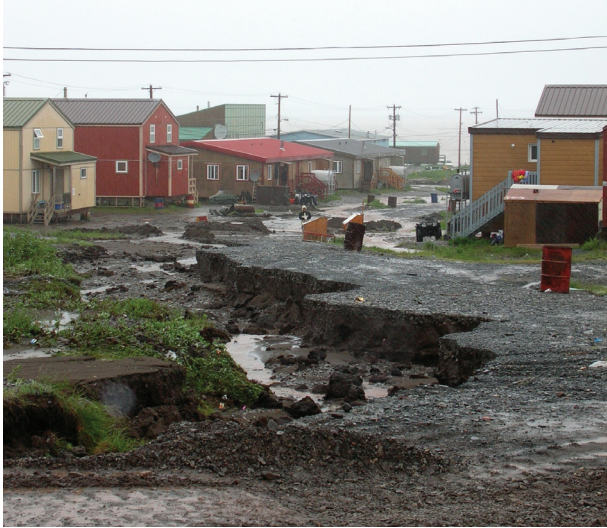
Fig. 5 Road and culvert erosion in Kugluktuk, NU, following a storm on 20–21 July 2007.
